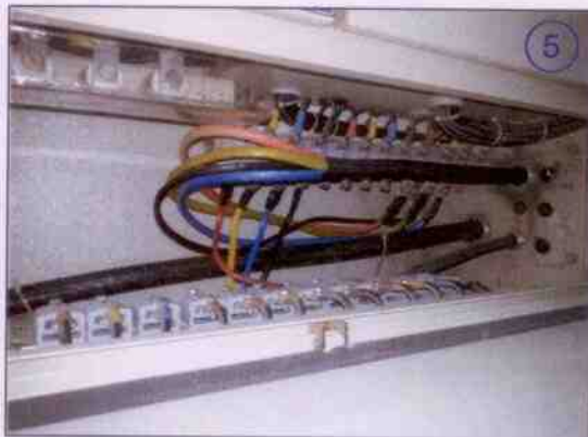
OUTGOING CABLE ALLEY
