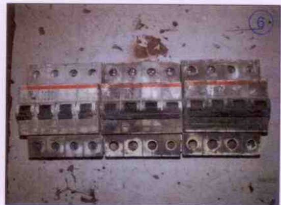
DAMAGED MCB FRONT VIEW
