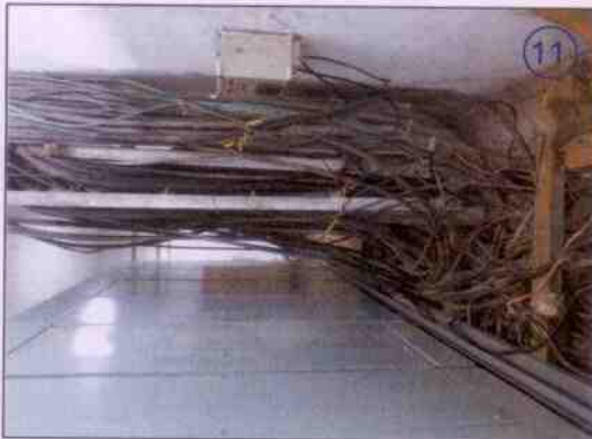
CABLE DRESSING REQUIRED
