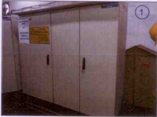
POWER DISTRIBUTION BOARD - 2
