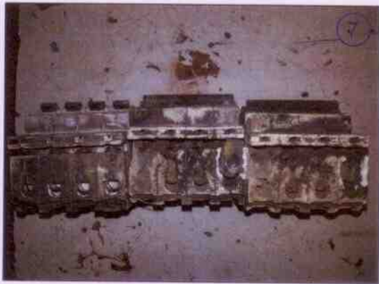
DAMAGED MCB INCOMING SIDE VIEW
