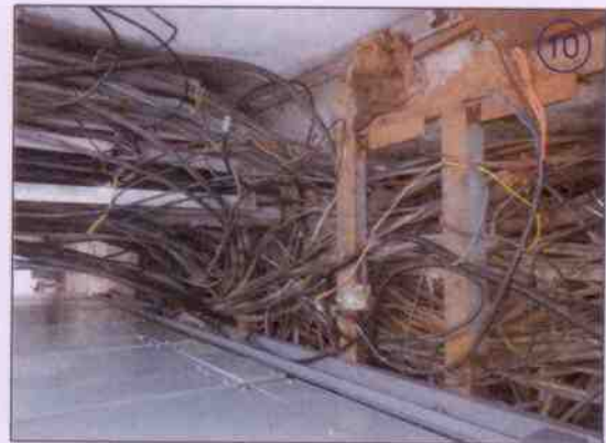
CABLE DRESSING REQUIRED
